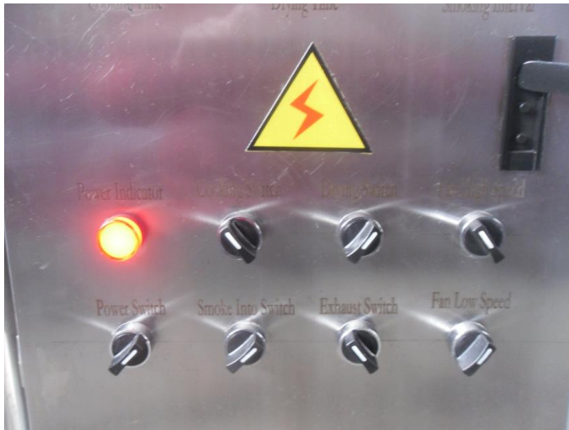
When the smoke switch display
